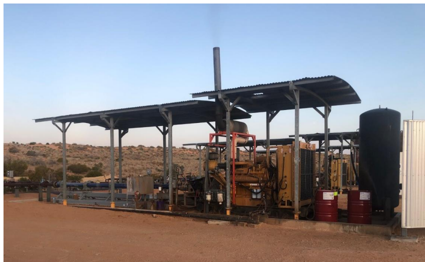
Photo 3: Worrior HPS 3 jet pump power fluid pump
