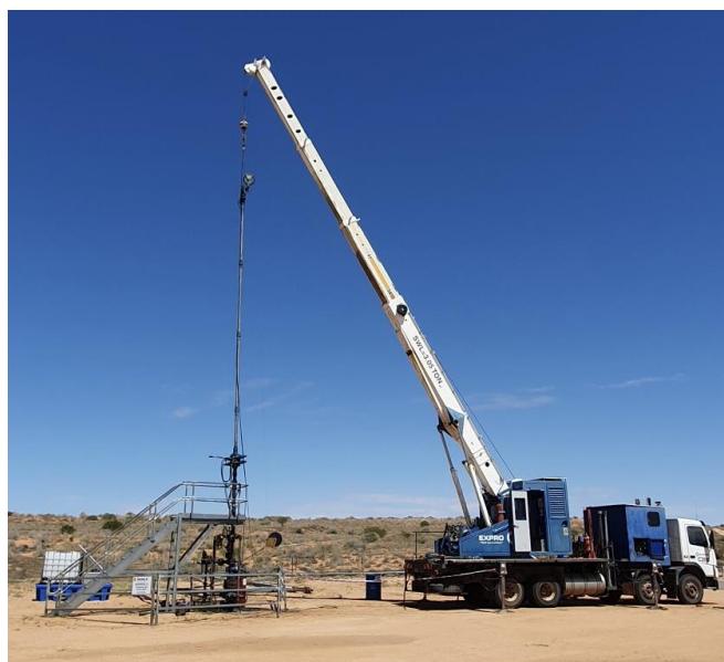
Photo 1: Slickline unit operating in the Worrior field
